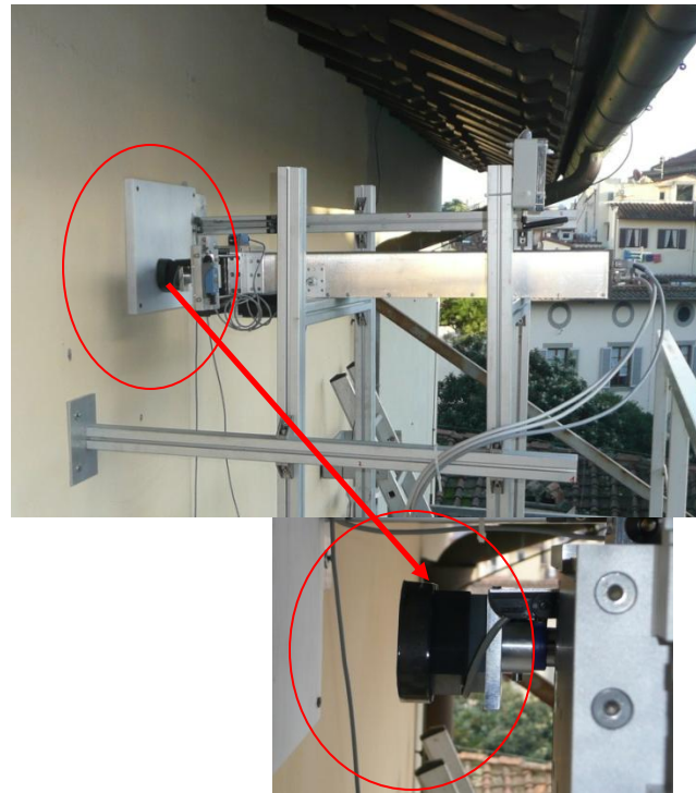
SENSOR INSTALLED ON THE ROOF OF MUSEUM OF THE CATHEDRAL SANTA MARIA DEL FIORE - FLORENCE, ITALY
